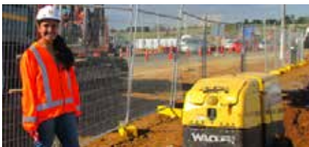
Sapoa Rimoni NZDE (Civil) Manukau Institute of Technology Site Engineer, Hawkins Infrastructure
